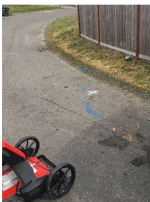
X marks the spot: Field technicians locate pipes using GPR. The "X" marks the suspected leak location.
