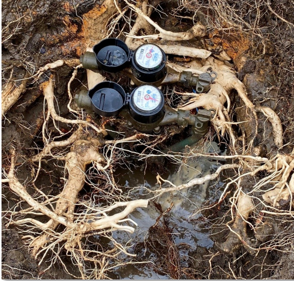
A meter box surrounded by tree roots.
