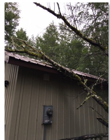
Tree damage at the Lew's 81st water system due to a winter storm
