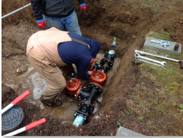
The PUD crew performing work at a water system in Thurston County.
