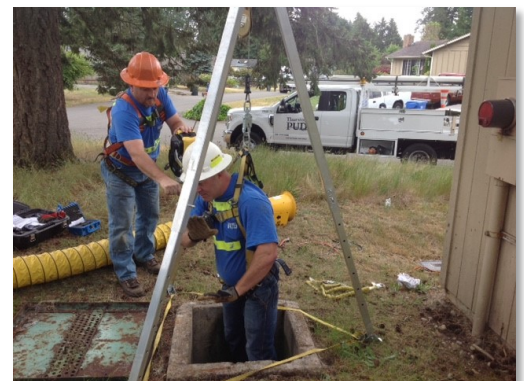
The PUD crew is shown using safety equipment to access an underground well at a water system in Pierce County.
