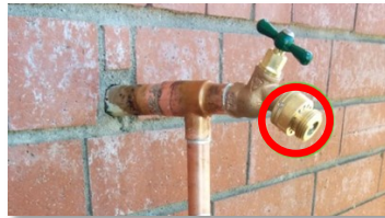
Above: Example of an atmospheric vacuum breaker (AVB)
