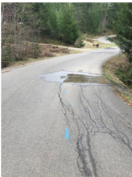
A large puddle on a dry road, caused by a mainline leak.
