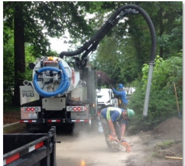
A PUD crew working to repair a water leak, classified as a repair. Taken in 2018.
