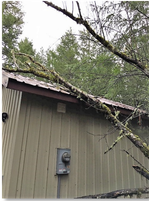
Pumphouse damage at a water system in Thurston County after a wind-storm.
