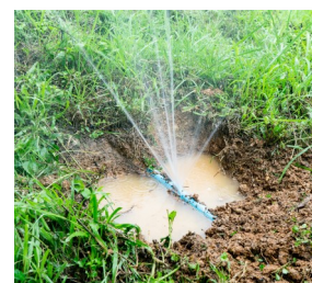
Example of a leaky customer service line
