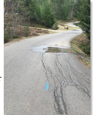
A large puddle on the road caused by leak.
