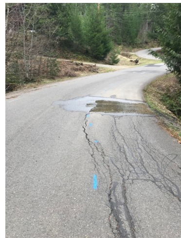
A large puddle on the road caused by a leak.
