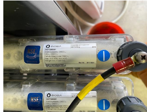
CL Generator Cells
