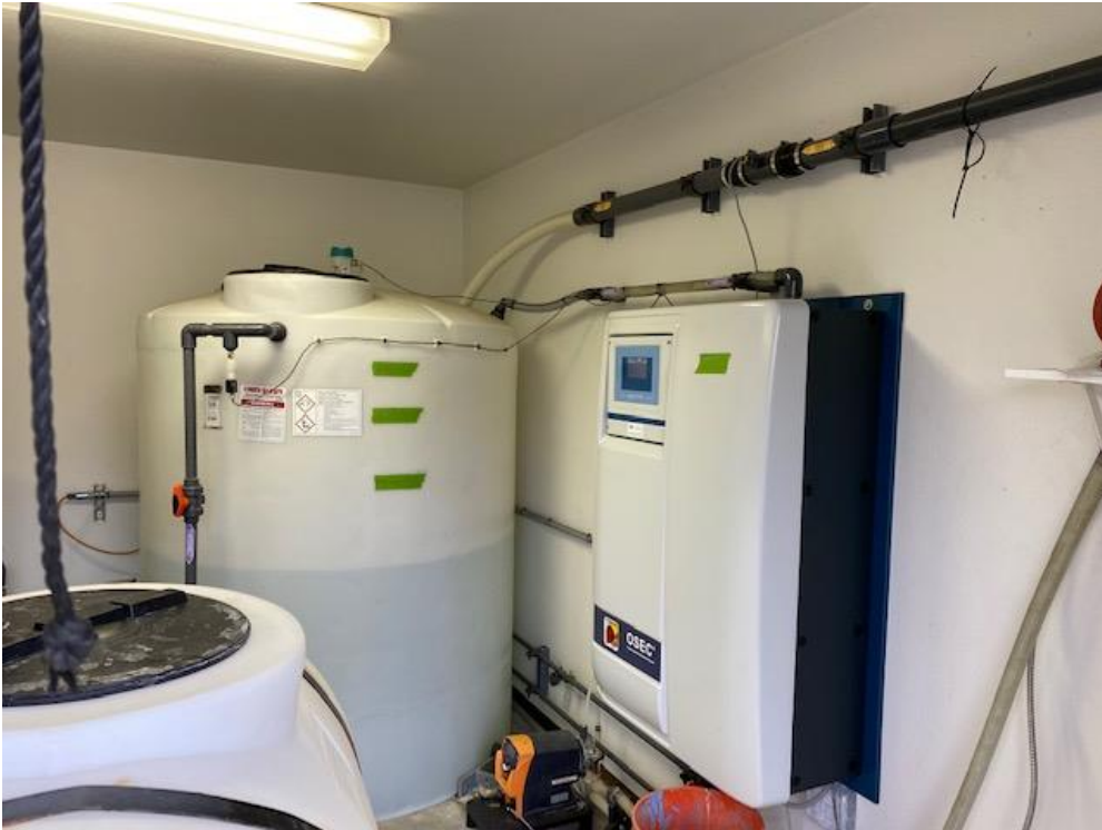
CL Generator and Storage Tank
