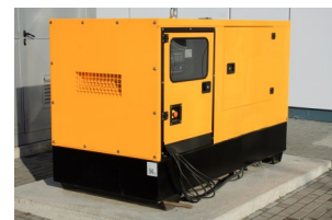
An example of a generator.
